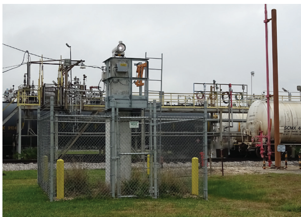
An OPSIS fence-line system installation
